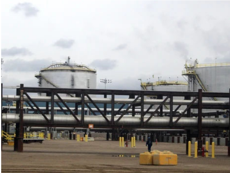
A worker walks beneath pipes at the Fort Hills oilsands project on Monday, September 10, 2018. Photo by Vincent McDermott /Postmedia
