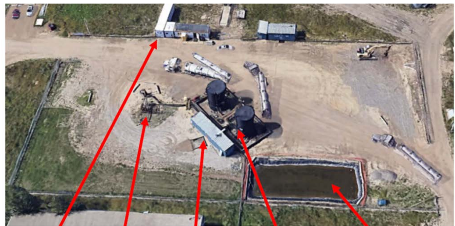
Offices 11-17 Wellhead Storage 2 750-barrel Tanks within containment c/w Catch Pond c/w Liner
